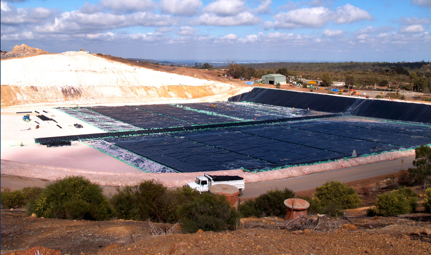
Lining a landfill at Red Hill Waste Management Facility. Image courtesy of Eastern Metropolitan Regional Council.
