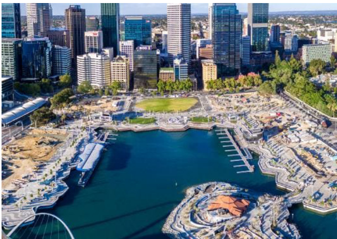
The site of the Elizabeth Quay is one of 23 unlined former waste dumps dotted around the Swan River. Picture: Michael Haluwana
